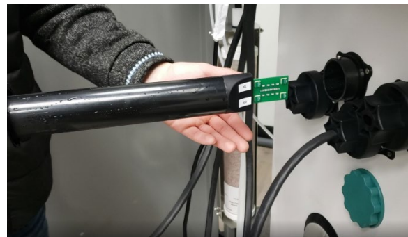
Figure 10: Electrical Twin Access Port
